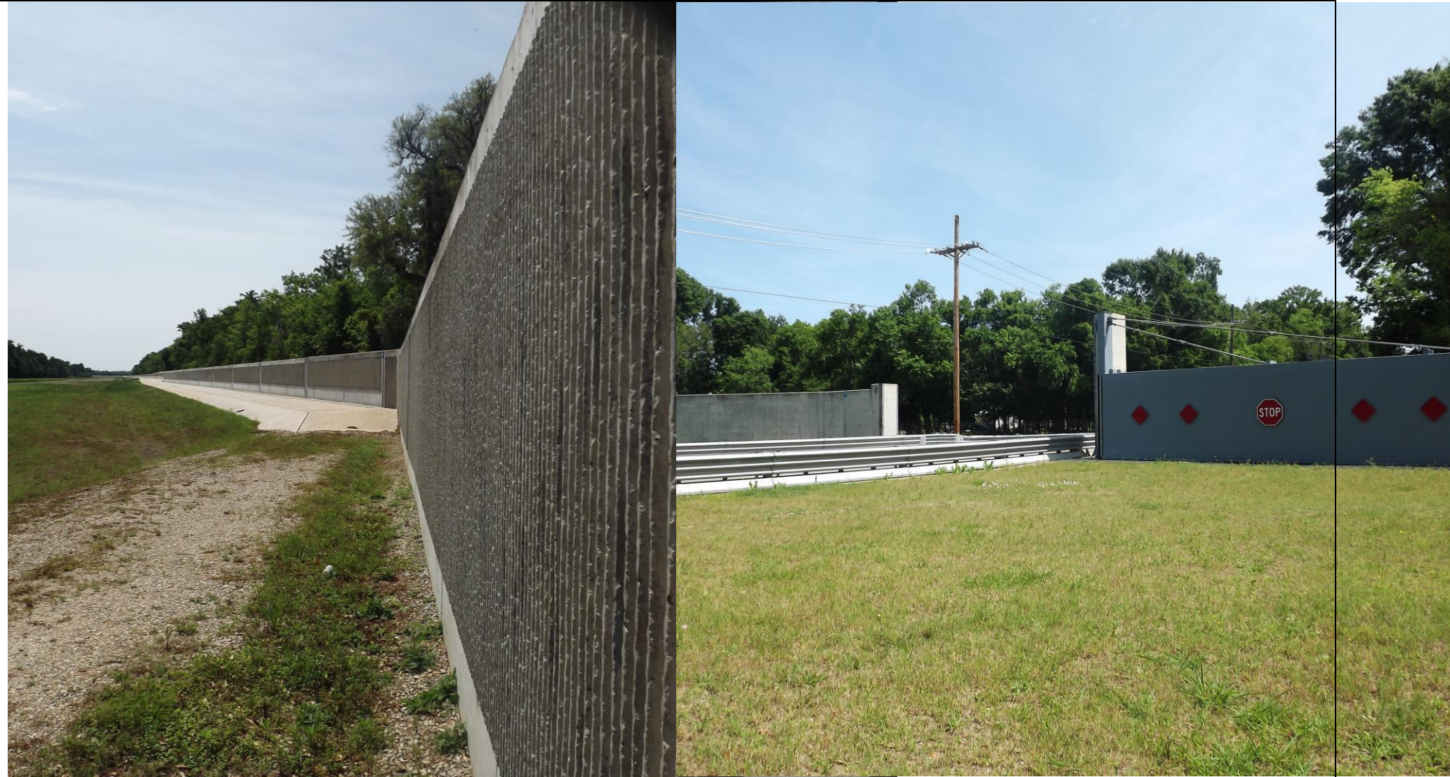
The Levee at Barataria Unit – new reinforced concrete walls to protect New Orleans from storm surges and flooding
